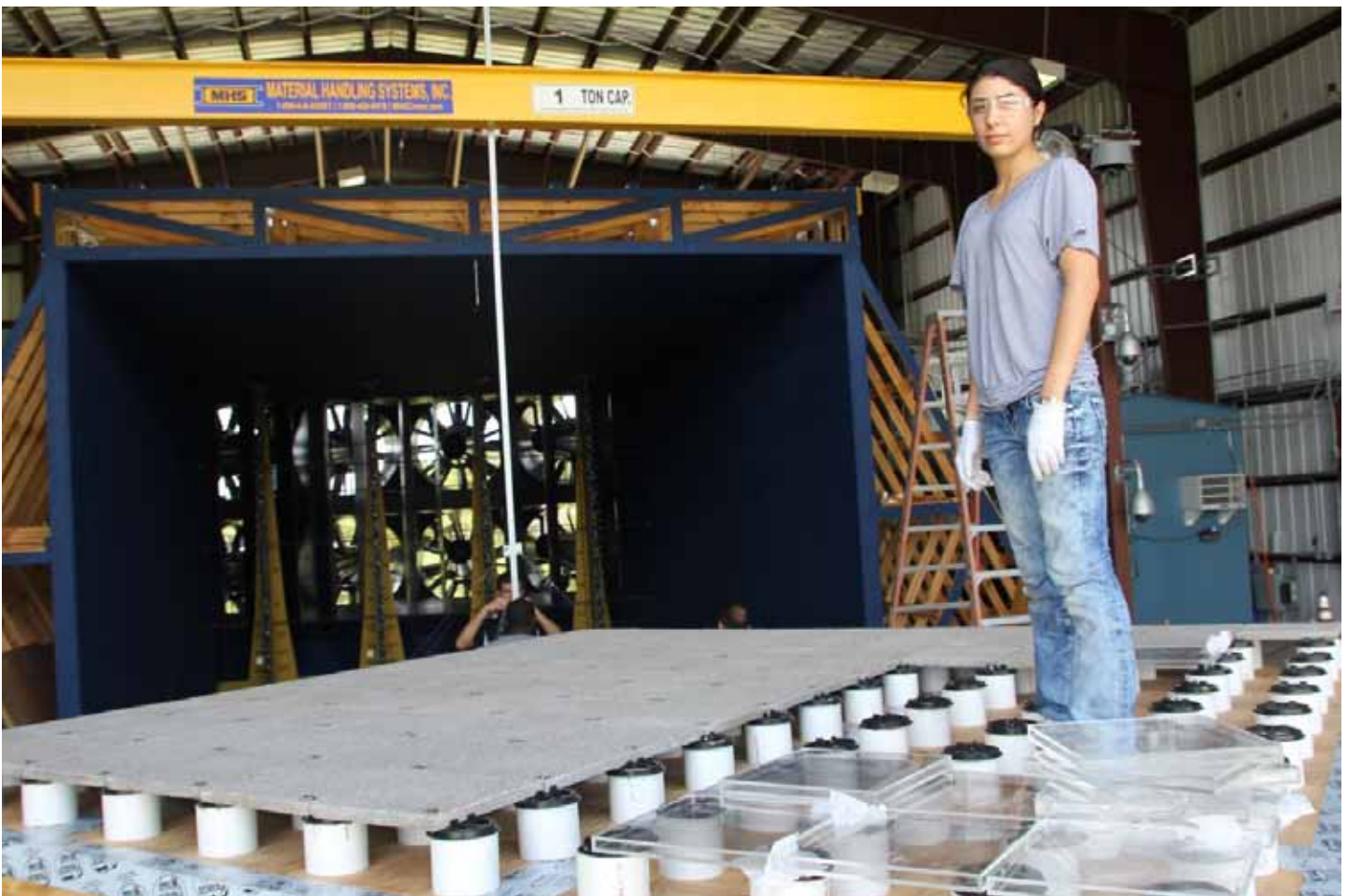
Maryam Asghari Mooneghi installing roof pavers for large scale wind testing at the Wall of Wind facility, Florida International University.
