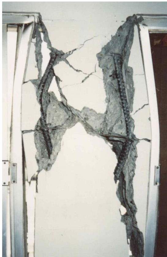
Figure 8. Shear failure and buckling of column
