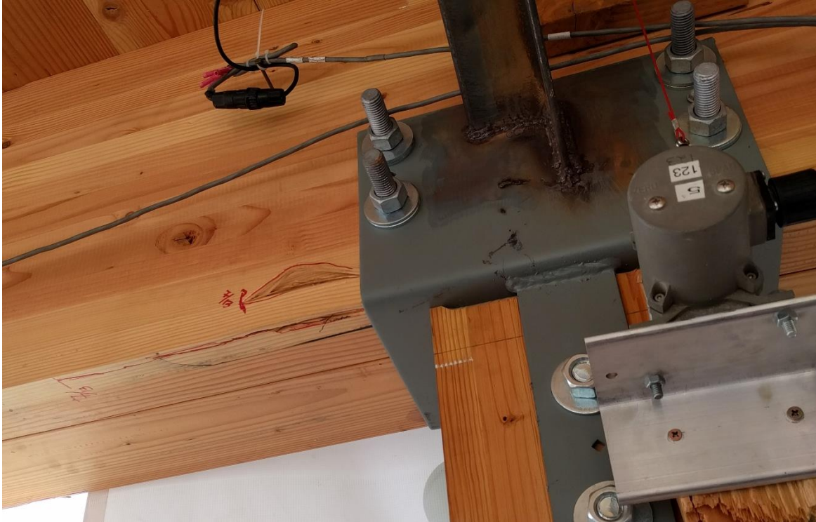
Figure 4. Small splinter of the beam near the connection (Same damage documented in figure 2)
