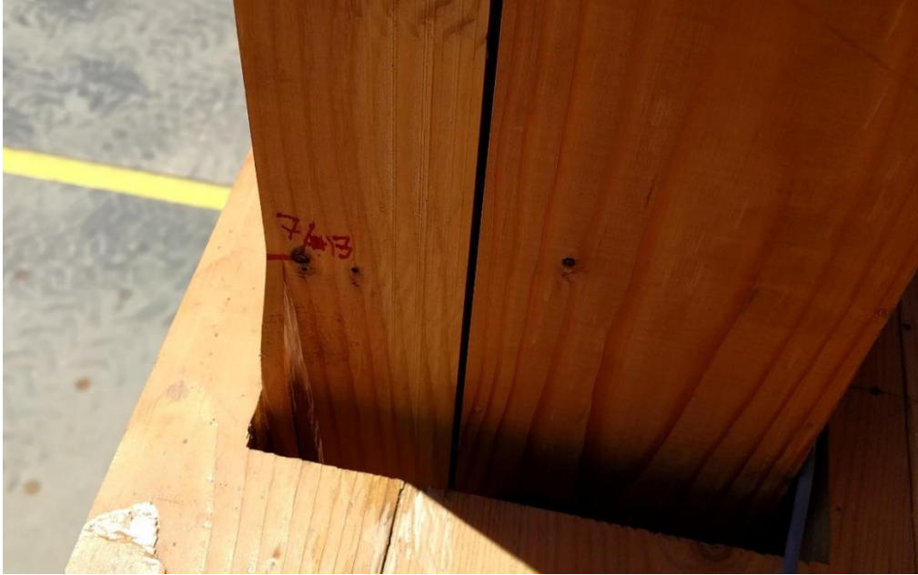
Figure 5. Wood splinter at the bottom of the discontinuous column and separation of the lamination located at the NW section of the second floor
