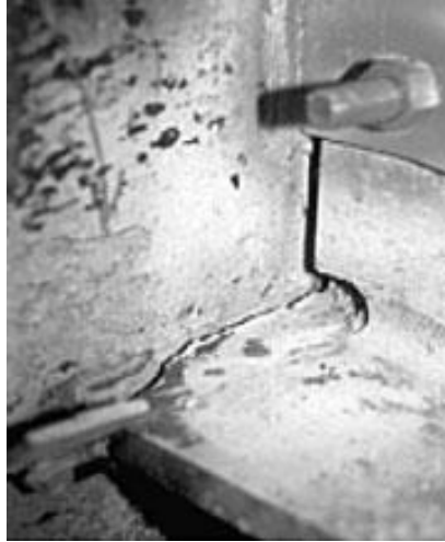
Figure 7. Weld cracking at the bottom of the flange
