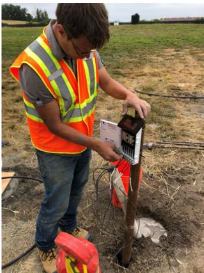
Dr. Leon van Paassen from the Center for Bio-mediated and Bio-inspired Geotechnics (CBBG) at Arizona State University installing a solar-powered wireless data logger for embedded sensors that measure hydraulic conductivity and water content of the soil in situ.
